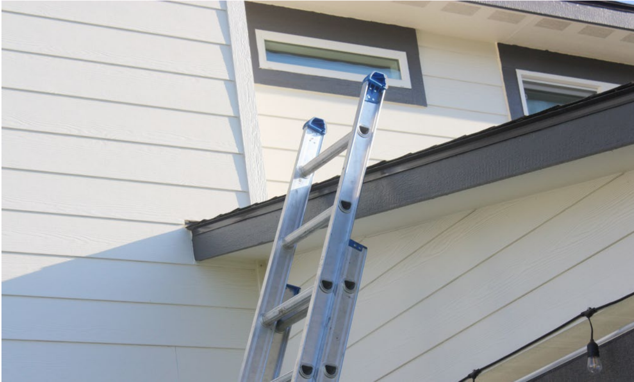
Photo 1. The ladder the installer used to climb onto the patio roof in order to pry on the edge of the upper roof.
