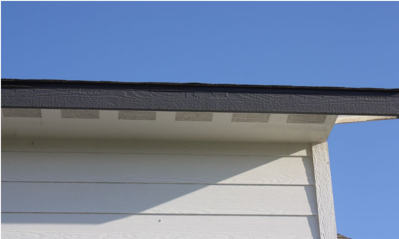
Photo 2. Upper roof above the patio where the installer was prying when he fell.
