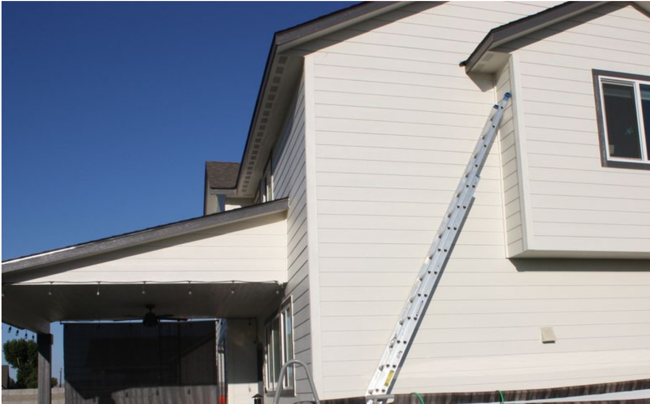
Photo 3. Edge of the patio roof where the installer was working and from where the fell, opposite from where the ladder was propped.
